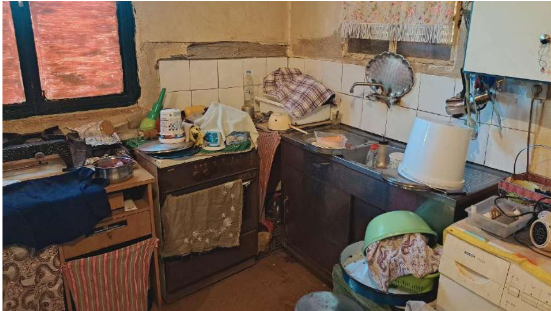
Figure 4 The old appliances, worn-out cupboards and deteriorating walls suggest a daily life marked by deprivation and poverty, visibly reflected in the condition of the kitchen.
