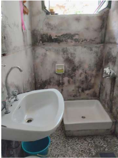
Figure 9 A bathroom showing clear signs of damp and mould, significant damage and conditions that make it difficult to maintain adequate hygiene.
